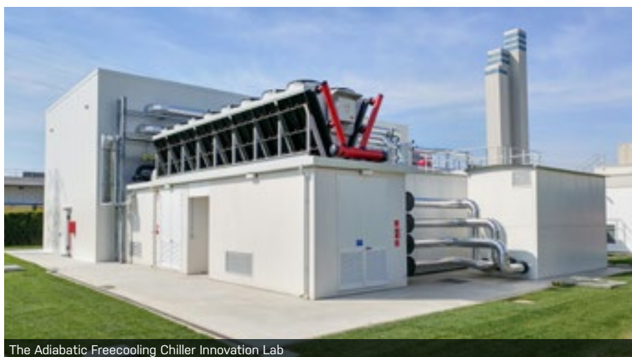
The Adiabatic Freecooling Chiller Innovation Lab
